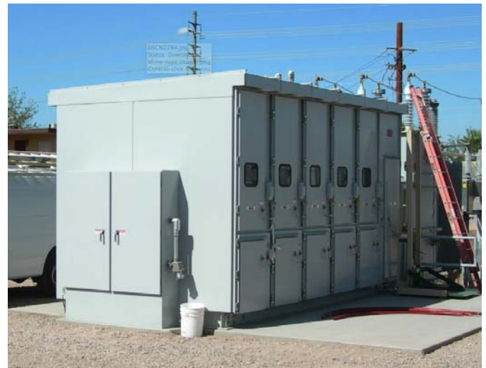
Figure 10. A small bank of medium voltage switchboxes.
