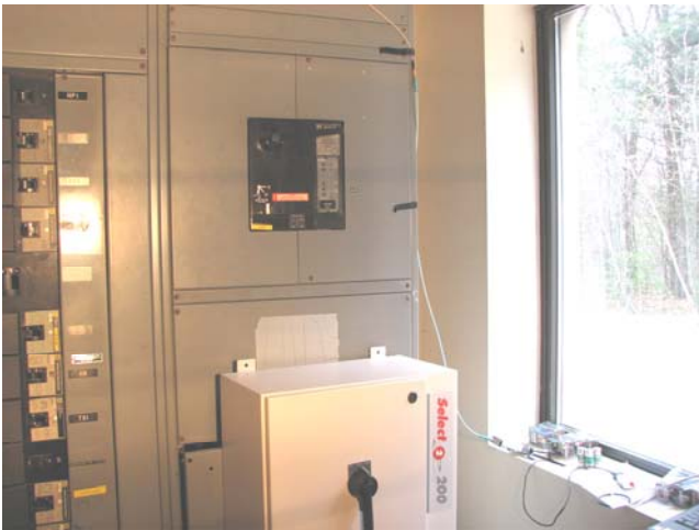
Figure 7: This picture shows the low voltage (408V) switchbox that was used for studying system installation issues.
