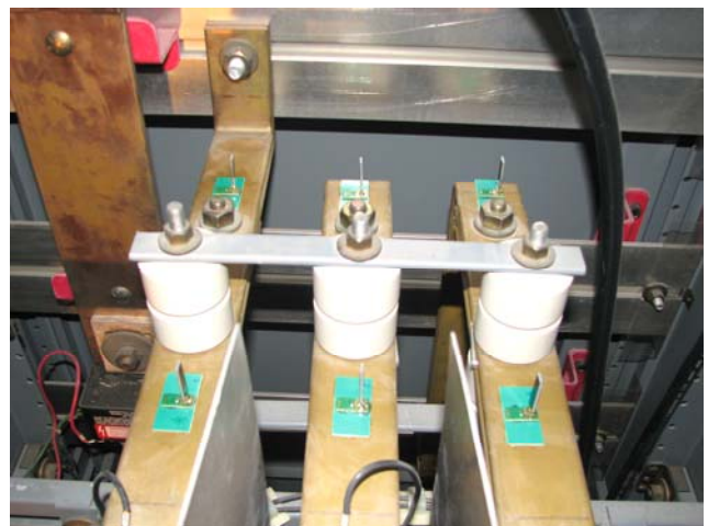
Figure 6. Installation in a low voltage switchbox. The upper picture shows installation on or near the switch contacts, using high temperature cable ties to secure the temperature sensing elements. The lower picture shows sensor modules incorporating small monopole antennas, which are adhesively mounted near bolted connections.
